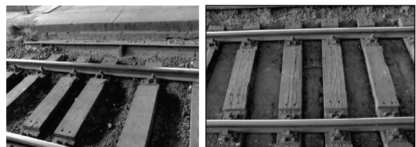
Fig. 5. Existing technical condition of the railway pavement: general view; Cross section through the span; lack of the prime of broken stone, moving undercut railway sleepers undercut and laying in wrong positions.
