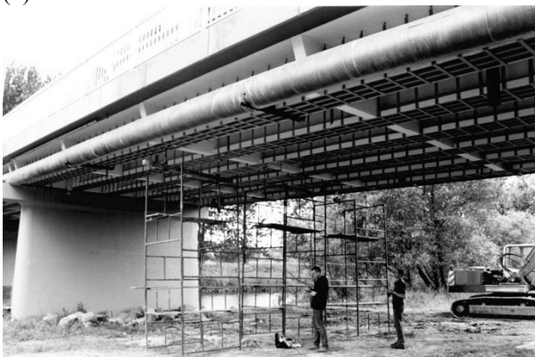
Fig. 1. General side view from the direction of the headwater of the road bridge: (a) localization of four trucks on tested span II (load scheme IIS) and (b) bottom view on the girders strengthening by CFRP strips.
