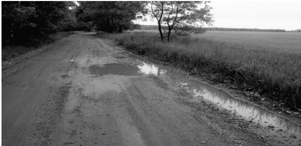
Fig. 6. Water amassing on the roadsides, lack of ditches on the sides [own photo].
