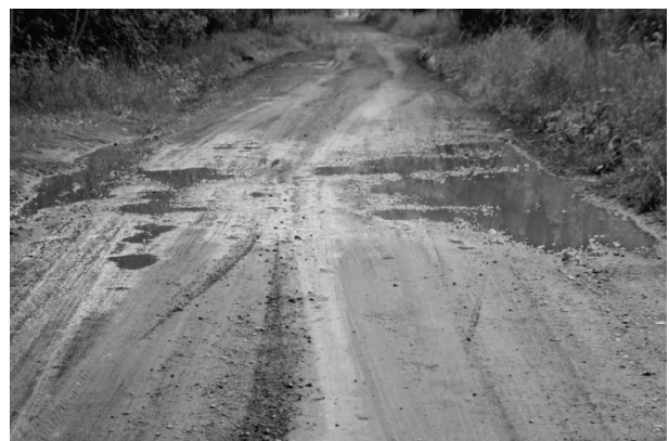
Fig. 4. Uneven structure of the surface, furrows and lack of water channelling [own photo].
