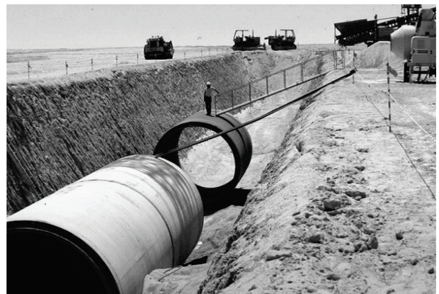
Fig. 3. 1,100 km long pipeline with a diameter of 4 m for transport of water across the desert in Libya.
